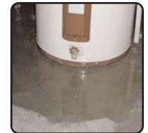
Flood Water Sensors
