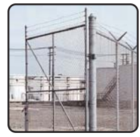
Perimeter Fence Vibration Sensors, Motion Sensors, Cameras
